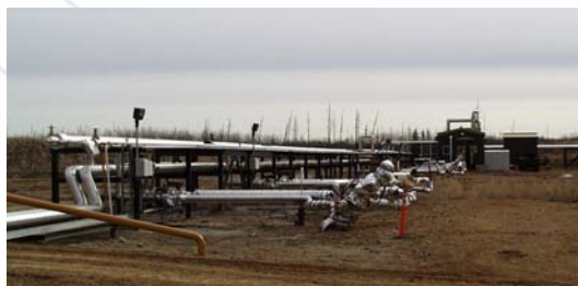
Dover Facility Well Pairs & Pipelines
